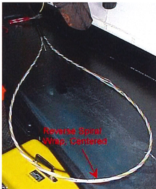
Figure 3: Exposed Mid-Sheath Buffer Tubes
