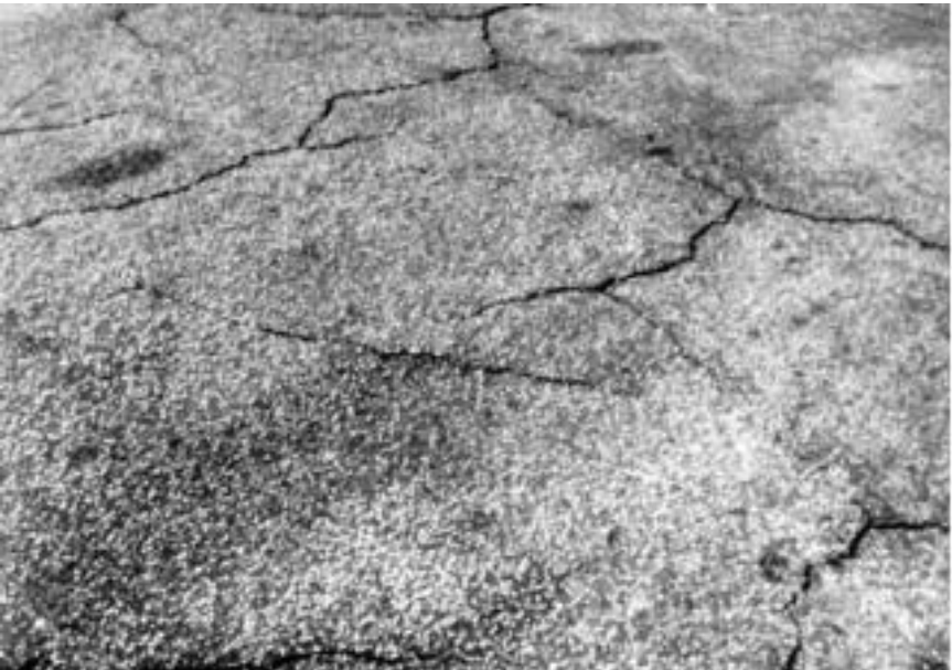
FIGURE 6: EXAMPLE OF BLOCK CRACKING (ASTM) This image is from the ASTM D6433 "Standard Practice for Roads and Parking Lots Pavement Condition Index Surveys." Block cracks are when pavement breaks into "chunks" or "blocks" that are roughly rectangular, caused by internal stress from temperature or lack of lateral support.
