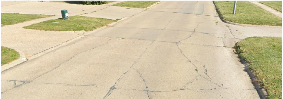
FIGURE 13: EXAMPLE OF “POOR” CONDITION PCC – E ASHLAND AVENUE E Ashland Avenue, west of N 5 th Street, has a CityPCI score of 32/100.
