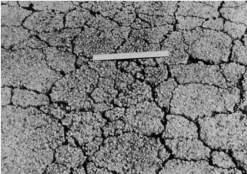
FIGURE 5: EXAMPLE OF ALLIGATOR CRACKING (ASTM) This image is from the ASTM D6433 "Standard Practice for Roads and Parking Lots Pavement Condition Index Surveys." Alligator Cracks are when pavement breaks into a "scaly" pattern typically caused by fatigue, either from repeated heavy loads, lack of sufficient subgrade support, or weakened material due to drainage issues.
