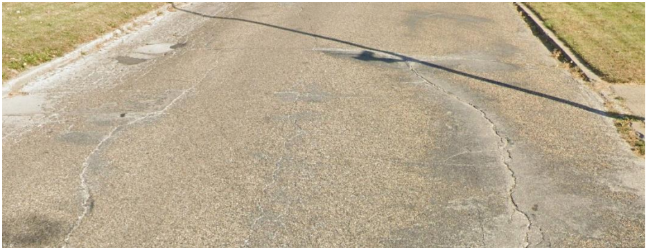
FIGURE 16: EXAMPLE OF “VERY POOR” CONDITION COM – N BUXTON ST N Buxton Street, just south of W Iowa Avenue, has a CityPCI score of 13/100.
