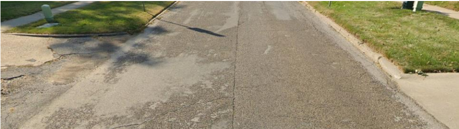
FIGURE 12: EXAMPLE OF “FAIR” CONDITION COM – N BUXTON STREET N Buxton Street, just south of W Henderson Avenue, has a CityPCI score of 45/100.
