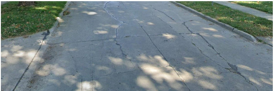
FIGURE 15: EXAMPLE OF “VERY POOR” CONDITION PCC – S 4 TH STREET S 4 th street, just south of E Salem Avenue, has a CltyPCI score of 9/100
