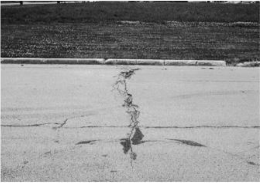
FIGURE 7: EXAMPLE OF TRANSVERSE CRACK (ASTM) This image is from the ASTM D6433 "Standard Practice for Roads and Parking Lots Pavement Condition Index Surveys." A common distress caused by a wide variety of issues.
