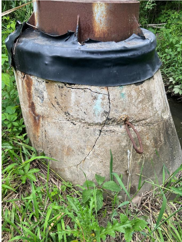
Cone Section Severely Cracked
