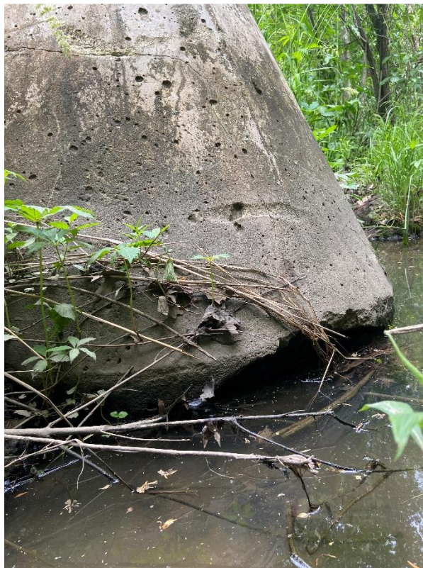
Part of Cone Section Missing near the Water.
