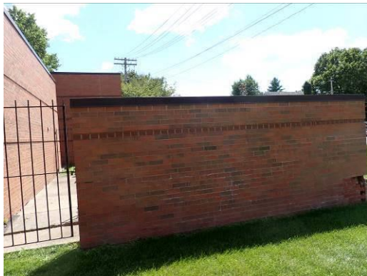
33, 34. Dumpster surround damage
