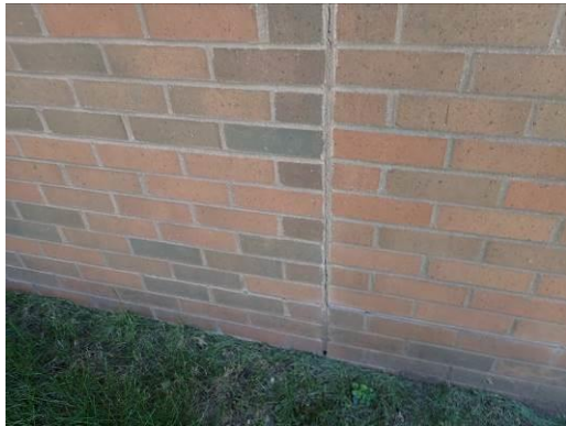
31. New joint sealant needed
