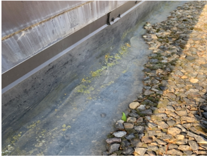
South wall starting to bridge out
