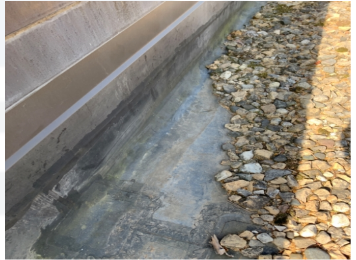
Another spot on south wall starting to bridge out
