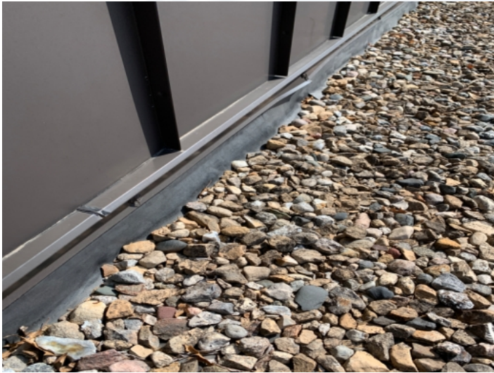
North wall starting to bridge
