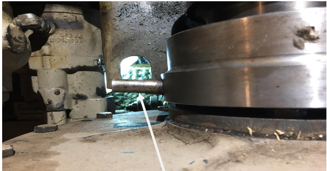
Both sides of piston support yokes on torque side are bent inward
