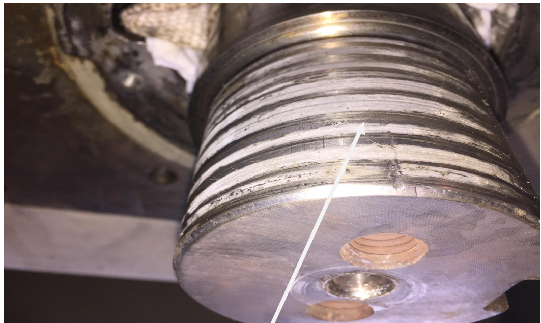
Hub shaft on gear box side is scored & possible stress cracking from sheared key
