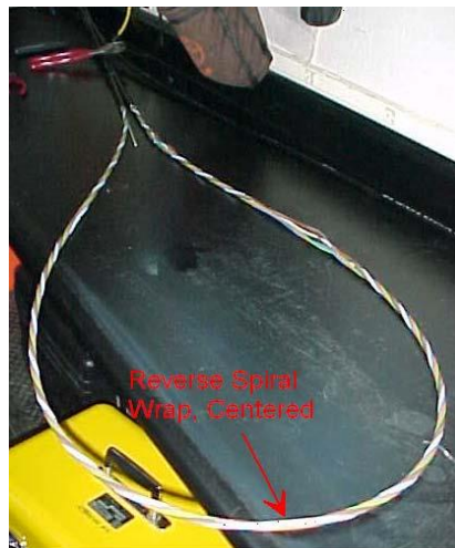
Figure 3: Exposed Mid-Sheath Buffer Tubes
