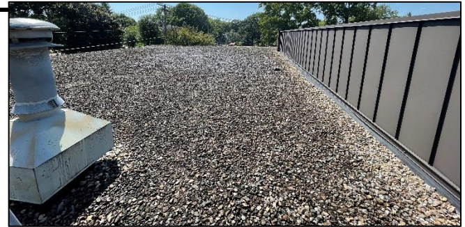
Standing water on roof
