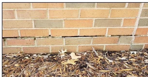
Deterioration of library exterior
