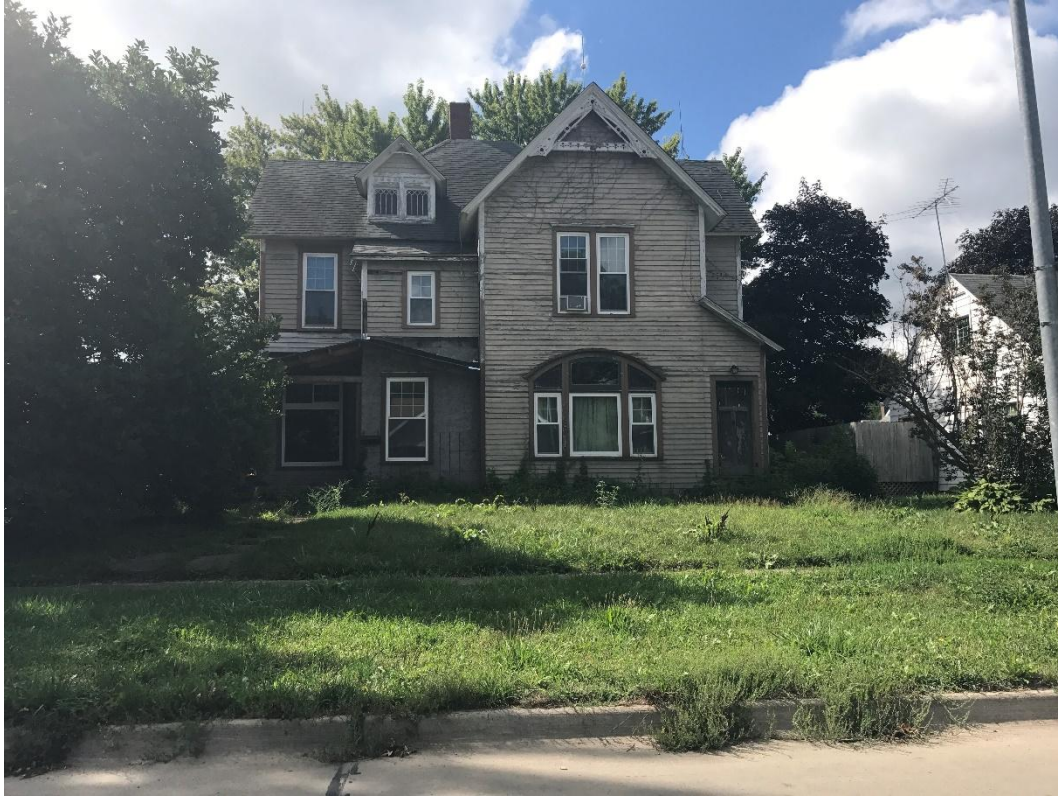
FIGURE 2 – EXAMPLE OF DETERIORATING STRUCTURE
