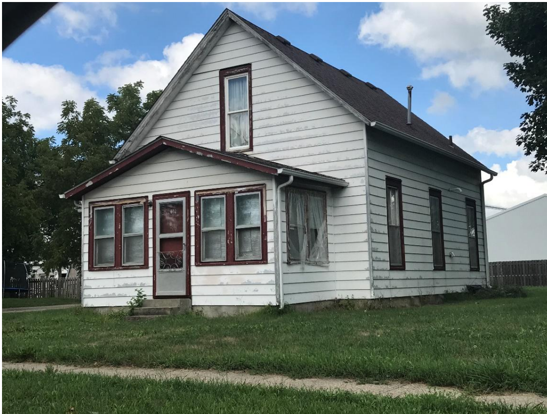
FIGURE 3 – EXAMPLE OF DETERIORATING STRUCTURE
