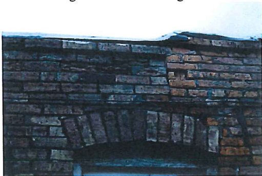
Photo 7485 Brick faces missing, mortar deteriorated.
