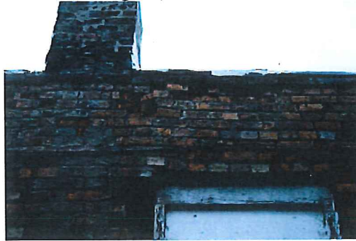
Photo 7476: Significant deterioration around the chimney area and continuing West.
