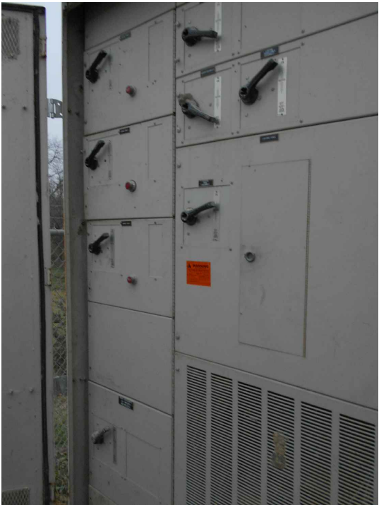
PHOTO 4 EXISTING MCC (OUTER DOOR OPEN)
