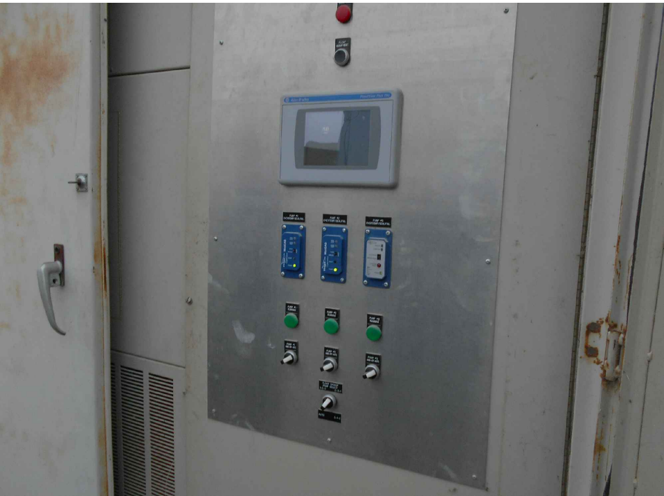
PHOTO 5 EXISTING CONTROL SECTION (OUTER DOOR OPEN)
